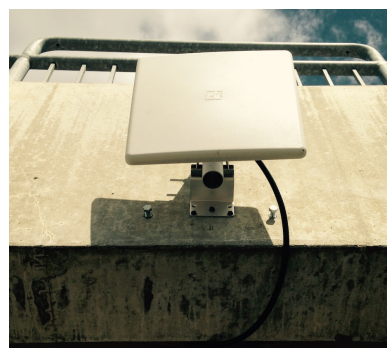
Figure 1. RFSN Antenna in Stadium
