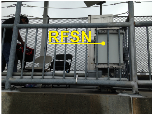
(b) RFSN Enclosure in Stadium
