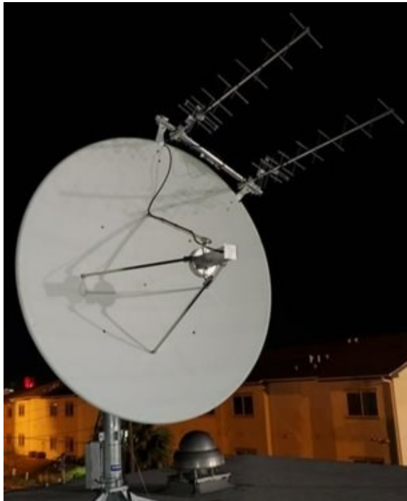
Figure 1: S-Band and UHF antennas on ground station roof
